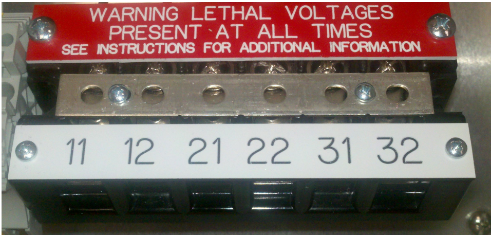
CT Connector Block with Shorting Screws Removed (Ready for Sensing)
