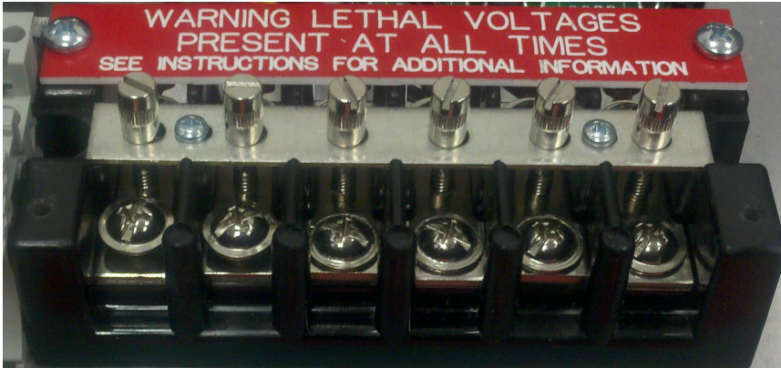
CT Connector Block with Number Plate Removed (Ready for Connection)
